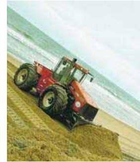
Beach replenishment work began in Dewey Beach on Tuesday, March 10. (John King photo)
